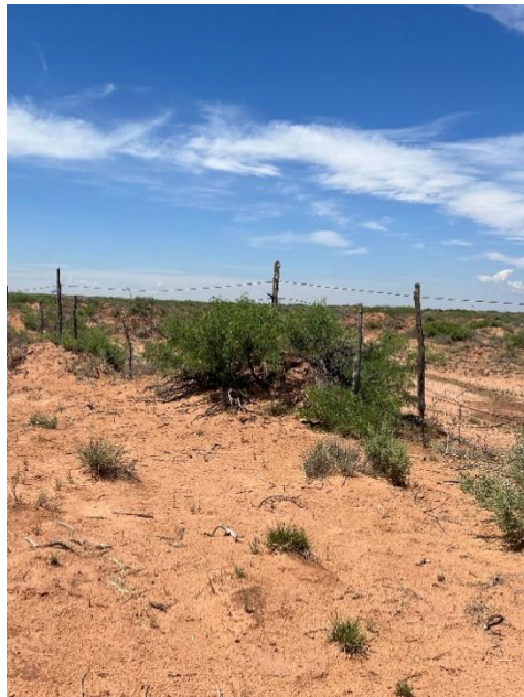
Figure 26. Dilapidated boundary fencing in need of replacement.
